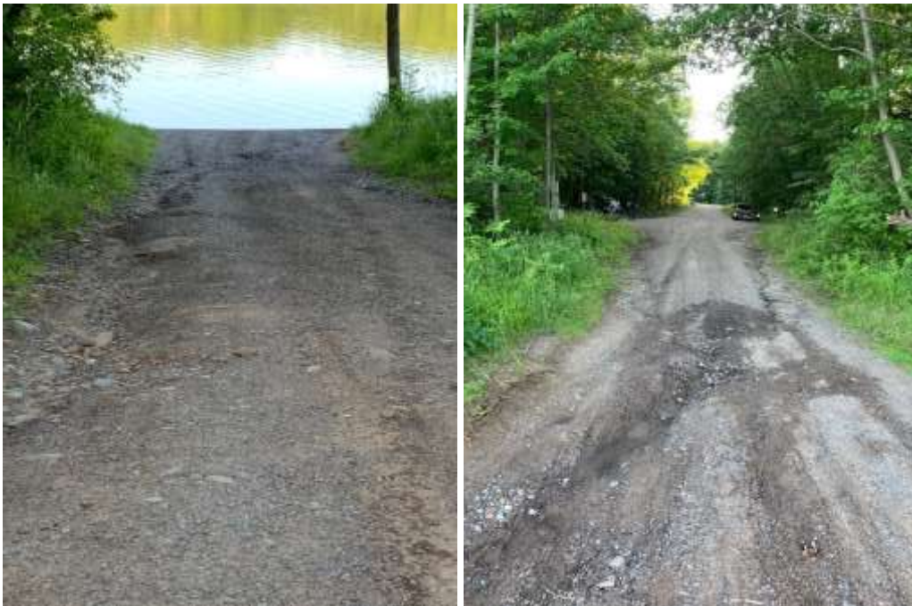
Figure 18: Erosion from the public boat landing facing the lake (left) and facing away from the lake (right)
