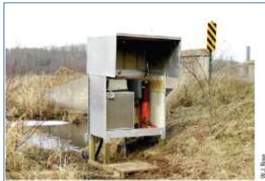
Figure 10 – Typical U.S. Geological Survey recording streamflow-gaging station with automatic water sampler for load determinations (Garn, Elder, & Robertson, 2003).
