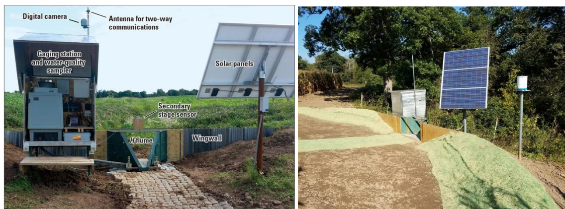
Figure 40: Example edge-of-field surface water monitoring station/system (left); actual Lake Redstone watershed edge-of-field monitoring station
