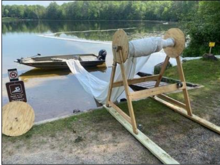
Figure 38: Limno-curtain material on a roll before installation (photo from Marinette Co. LWCD)
